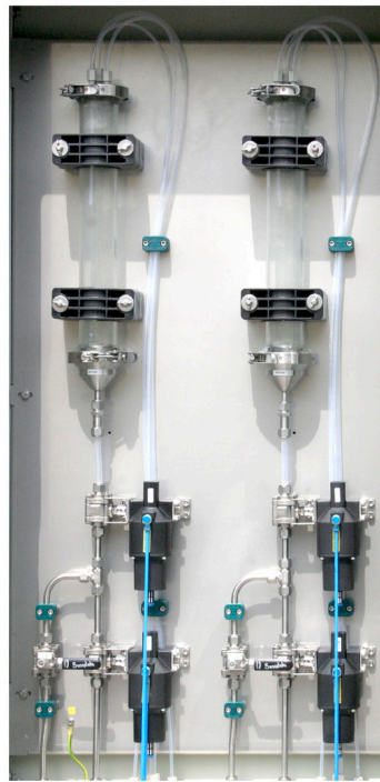
Customized preconditioning system on site
